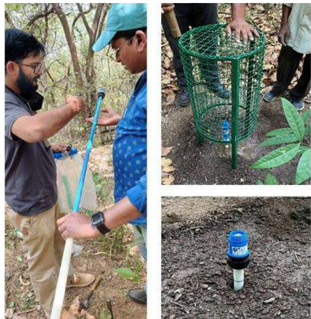
Fig. 20 Soil moisture sensor installation at Sanjay Van experimental site, New Delhi
