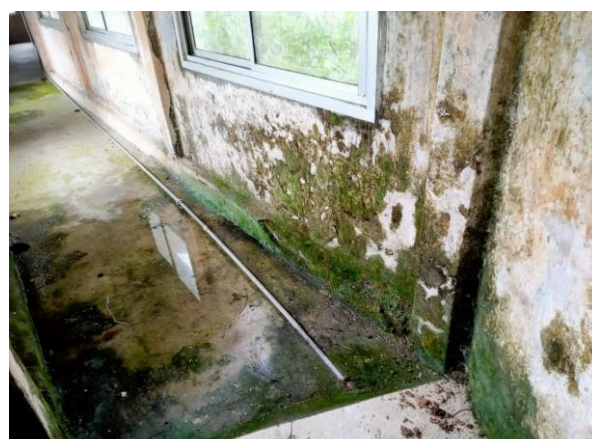
Passage require repair
