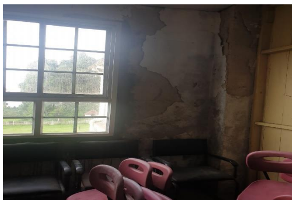
Utility Room require repair
