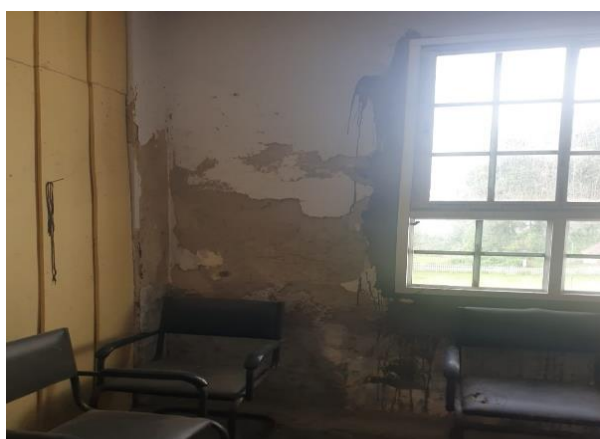
Damaged building Outer wall
