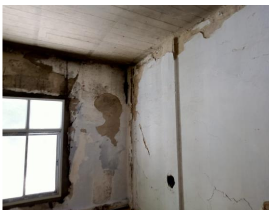
Damaged roof and wall
