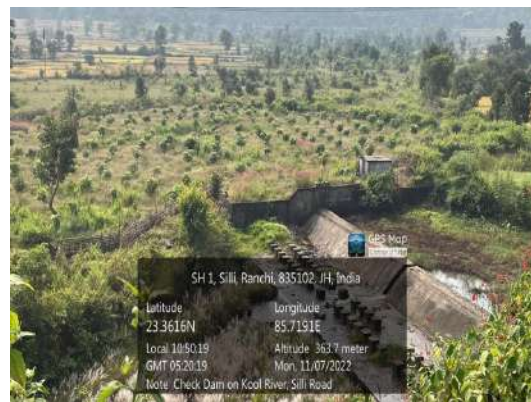
Figure.21: Check dam on Koel River, towards Muri Road. Mango plantation along river bank taken up by the farmers. Mango crop has been adapted by the farmers in different parts of Jharkhand, and Amrapali and Mallika variety is being practiced widely in this part.
