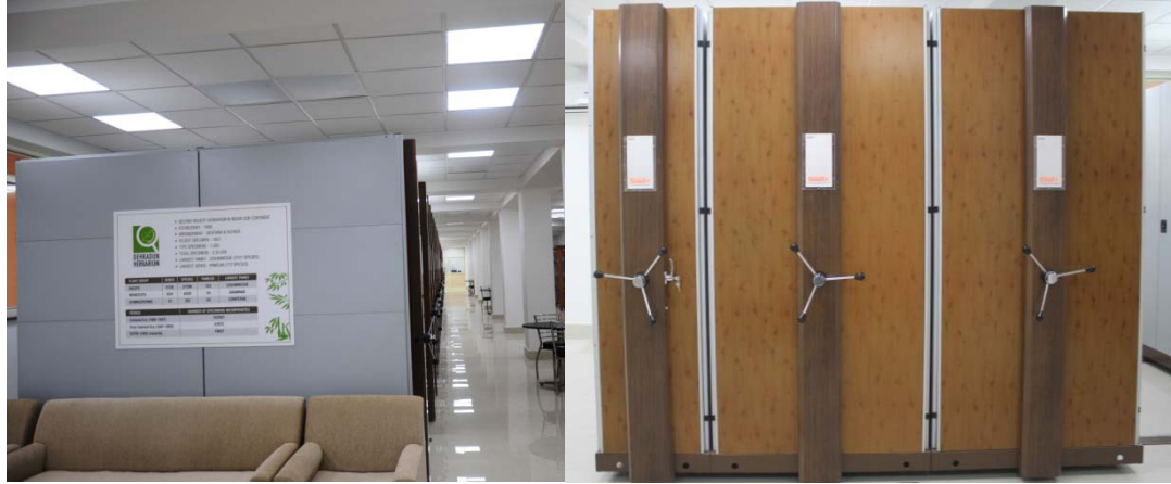
A view of New Herbarium hall with state of art Compactors after furnish
