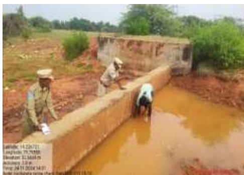
Check dam in Mittatmakur RF
