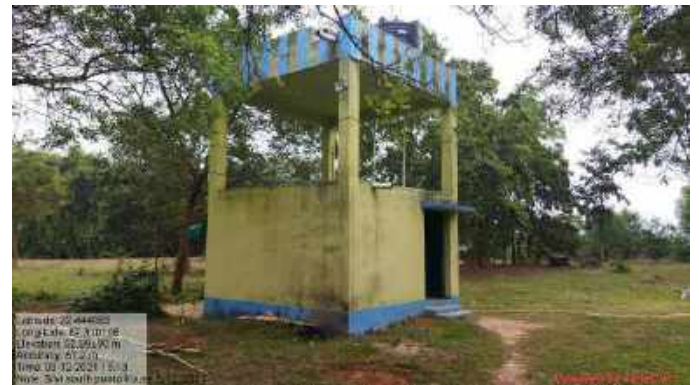
Pump house at modern nursery, Golapi Chawk, Medinipur
