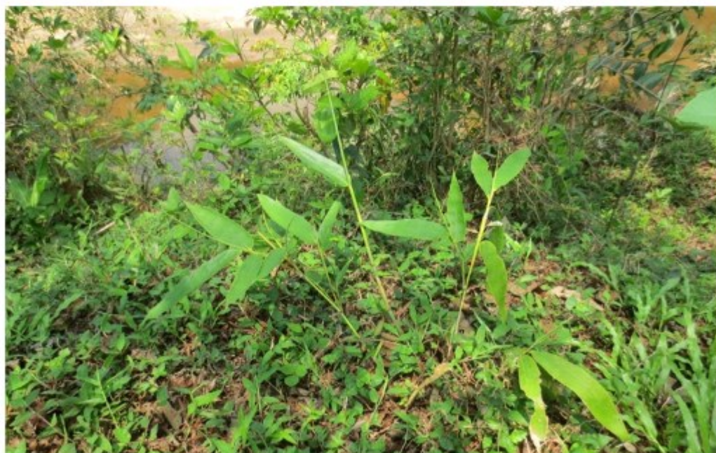
Current status of River Bank Stabilization activity from Rockwood kadavu to Anavattachira, at Mylamood Section, Kulathupuzha
