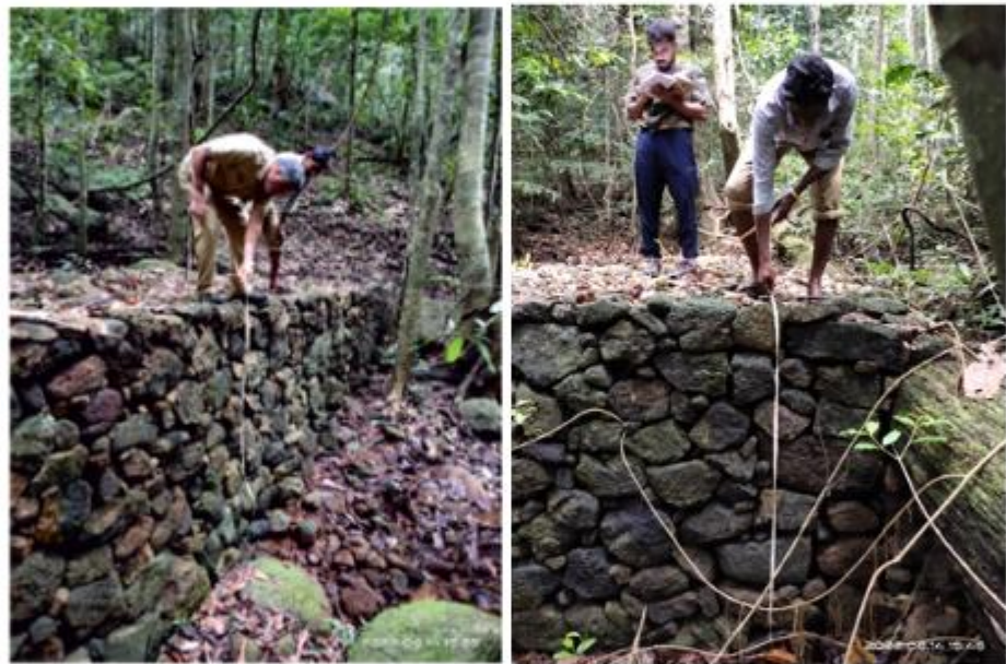
Gully plugging in four different locations
