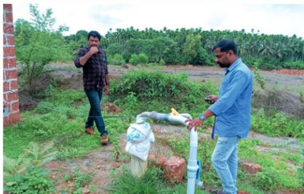
Drinking water facilities at Madaparambu
