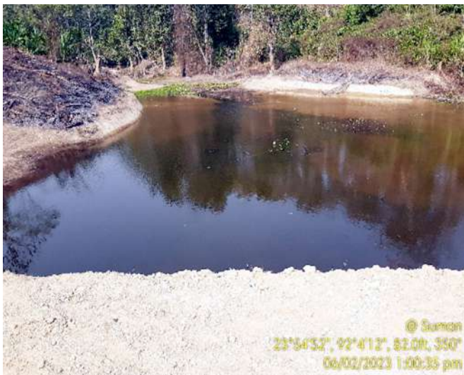
Check Dam construction under Amrit Sarovar Mission under CAMPA during 2022-23 at Labancherra VC
