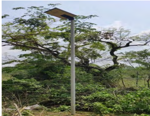
Installation of Solar Lights to reduce Human Elephant Conflict in areas prone to Human Elephant Conflict in Jhargram Division
