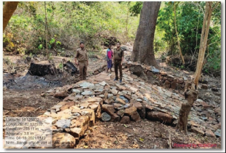
LBCD for Soil- Moisture Conservation at Mandra PRF under Jeypore Forest Division, Odisha
