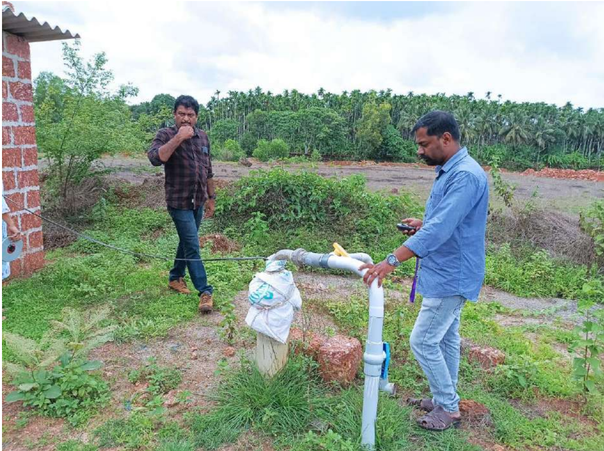
Drinking water facilities at Madaparambu
