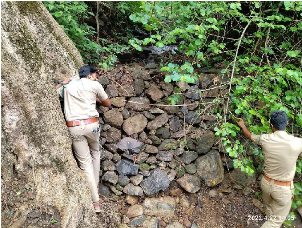
Gully plugging at Goodrickal
