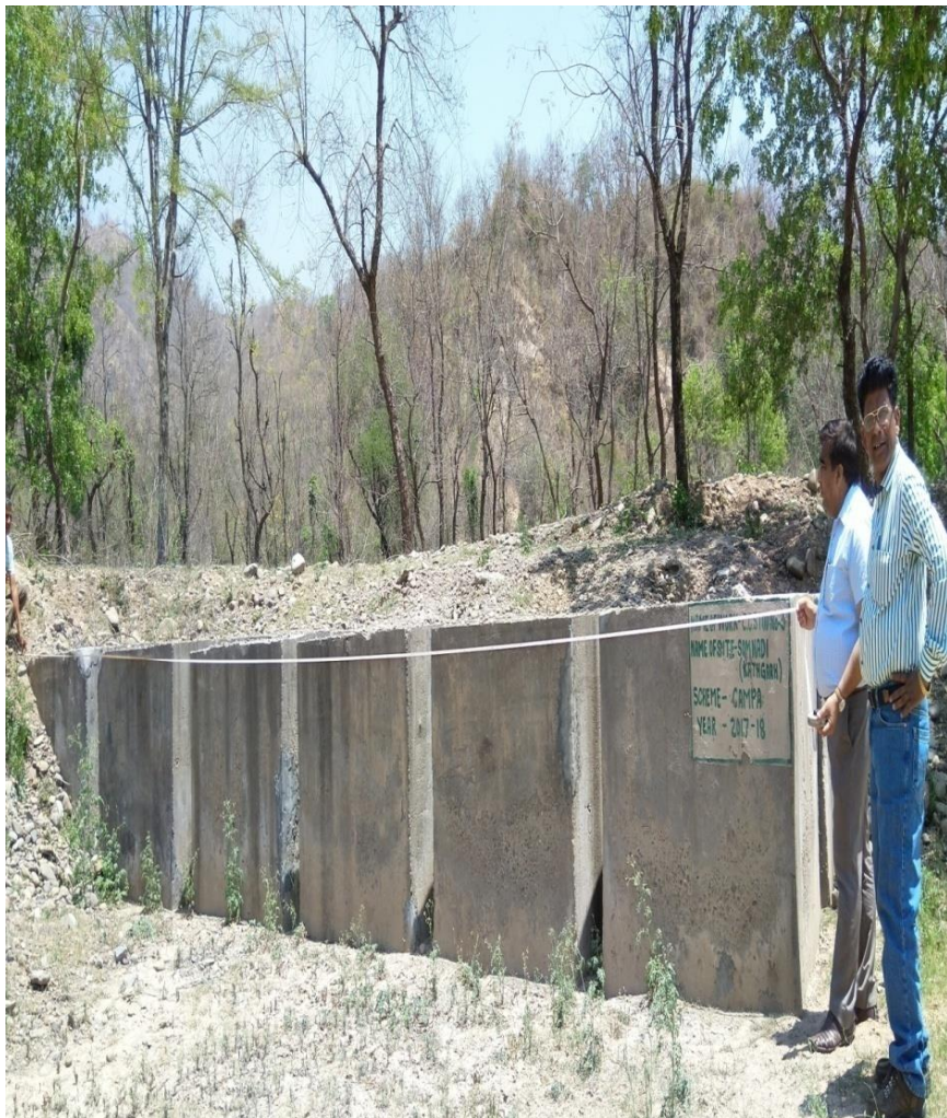
Division- Yamuna Nagar Wing- Territorial Year- 2017-2018 Range - Sadhaura Scheme- CAMPA Name of the component- Soil Conservation Work( C C Stud No.3 Name of the site- Kathgarh at Somnadi Target- C C Stud No 3
