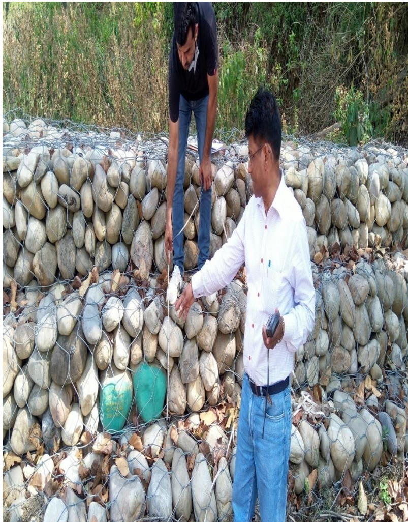
Division- Yamuna Nagar Wing- Territorial Year- 2017-2018 Range- Kalesar Scheme- CAMPA Name of the component- Soil Conservation Work Name of the site- Sukhrao River RIJ C- 16 Target- Crate Wire Structure No 5
