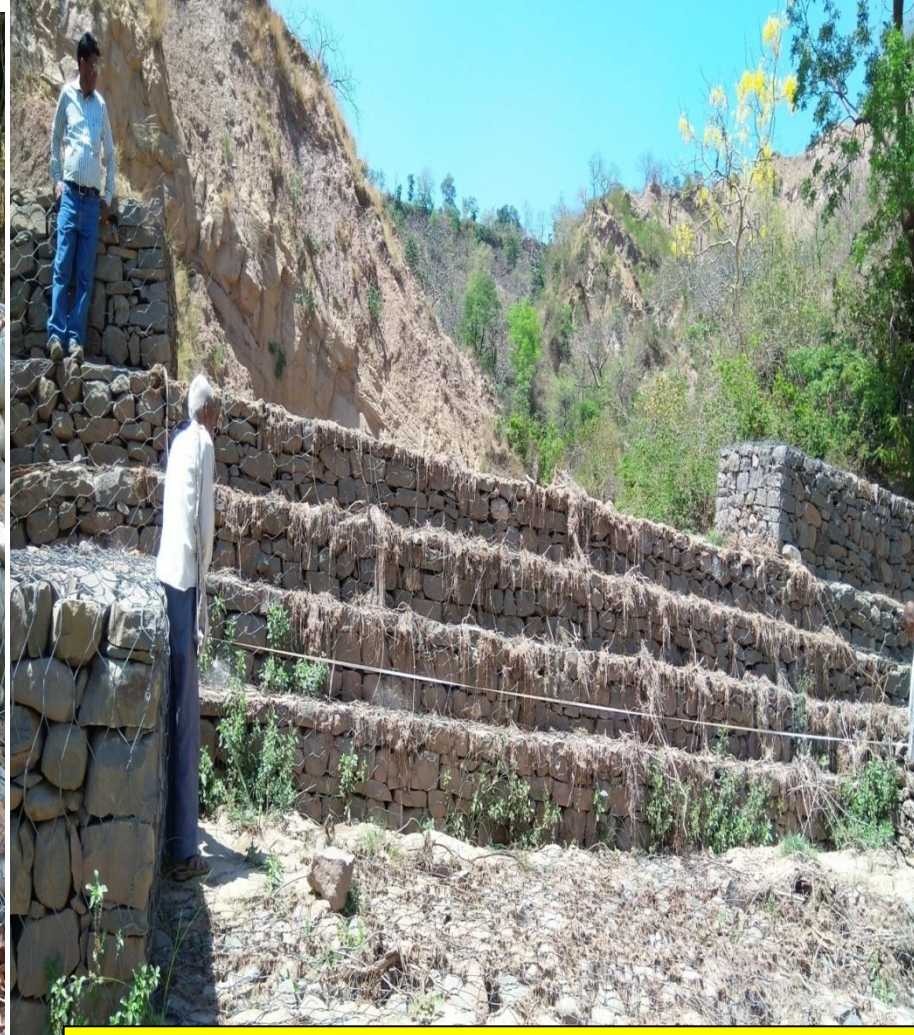
Division- Morni-Pinjore Wing- Territorial Year- 2017-2018 Range- Raipur- Rani Scheme- CAMPA Name of the component- Soil Conservation Work(Crate Wire Structure) Name of the site- Plasra ka Khala C-76
