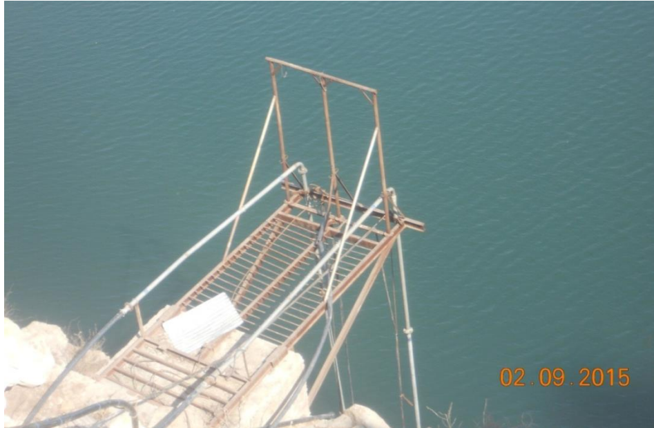
Irrigation system installed at the lake for irrigation of plantation
