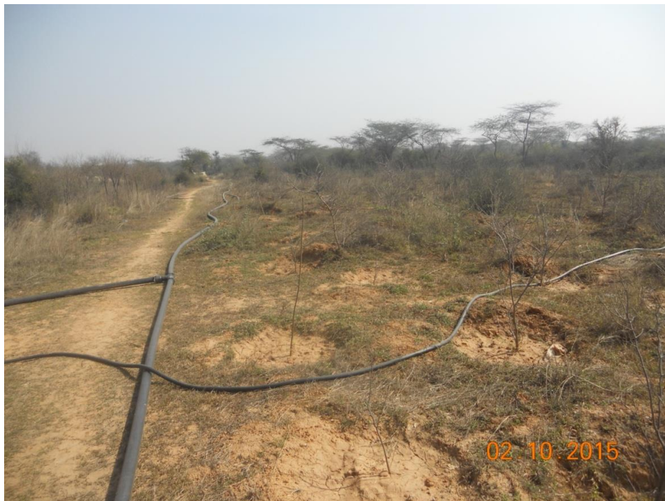
Pipe line for the distribution of irrigation water
